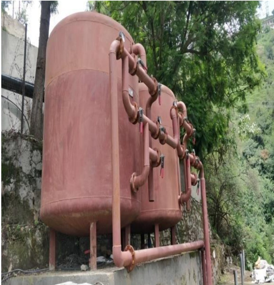
Dual Media filter installed for the removal of turbidity and suspended
