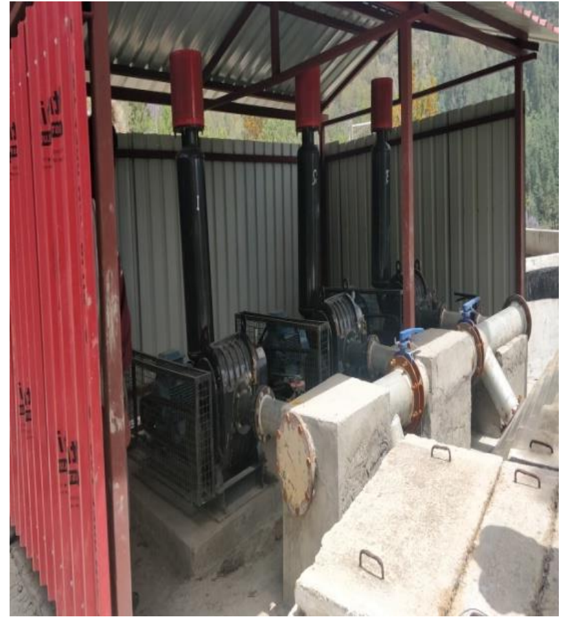
Diffuser system at STP Lalpani
