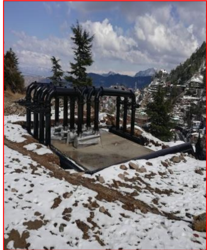
❑ UV system installed at Sanjauli
