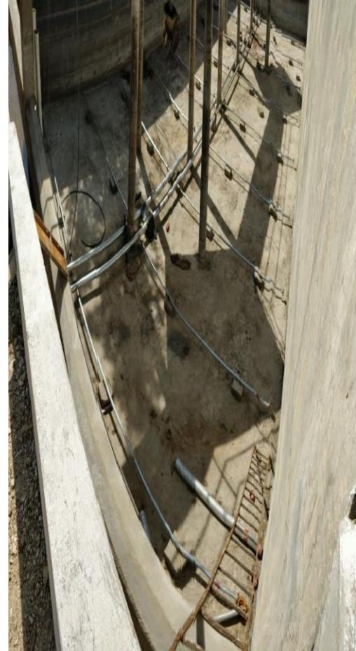
Aeration system installed at STP Malyana
